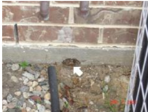
Post tension cable ends are exposed.
