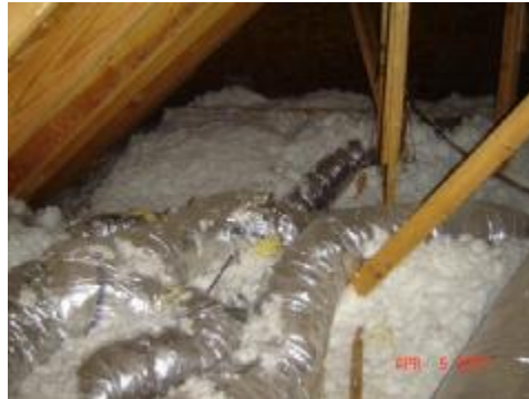
Ducts are on attic floor.
